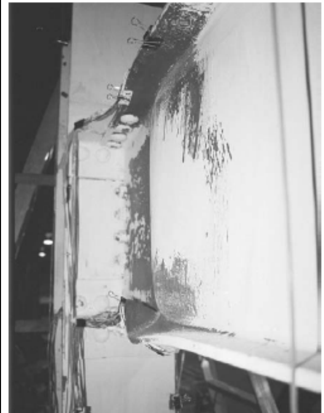
Figure 2-7. Web Local Buckling Limit State (SAC Project)
